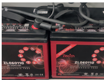
AGM batteries compartment
