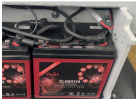
AGM batteries compartment.
